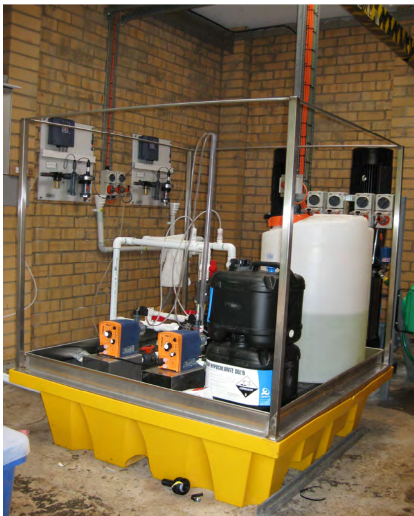
Figure 10: Jumbuk Water Supply Locality Remote Disinfection Site
