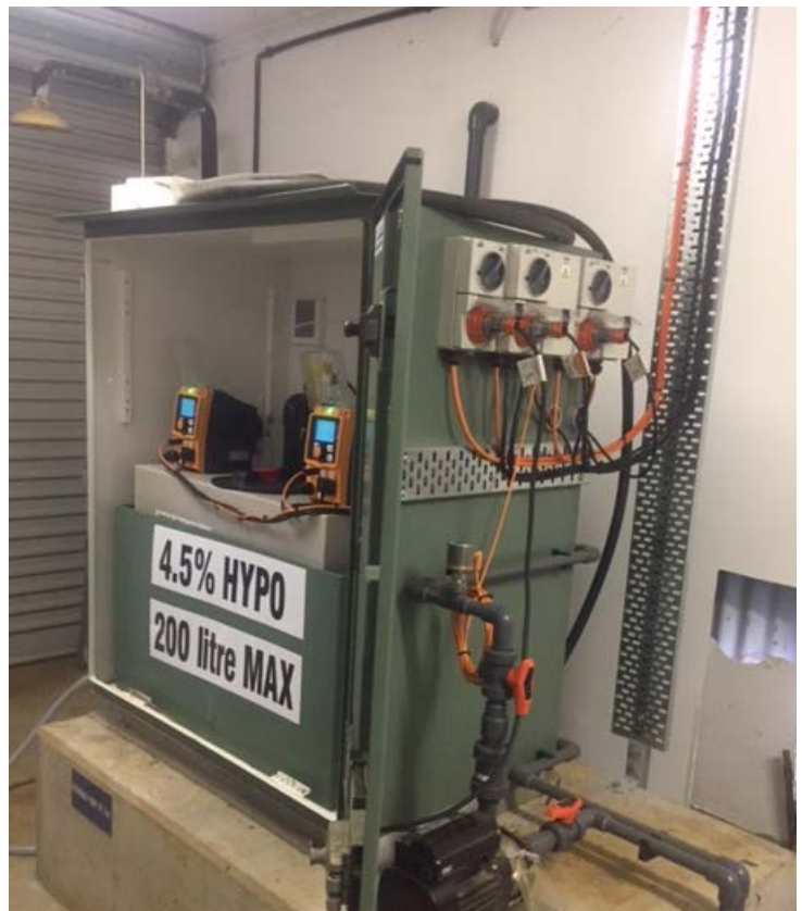
Figure 12: Thorpdale Water Supply Locality Project – Disinfection System Thorpdale water supply upgraded disinfection system for improved water quality and public health disinfection.
