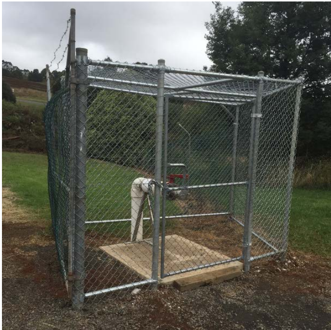
Figure 11: Thorpdale water supply locality project – Fill point upgrade Thorpdale Water Treatment Plant decommissioned and an improved water carting fill point installed for greater water supply security.
