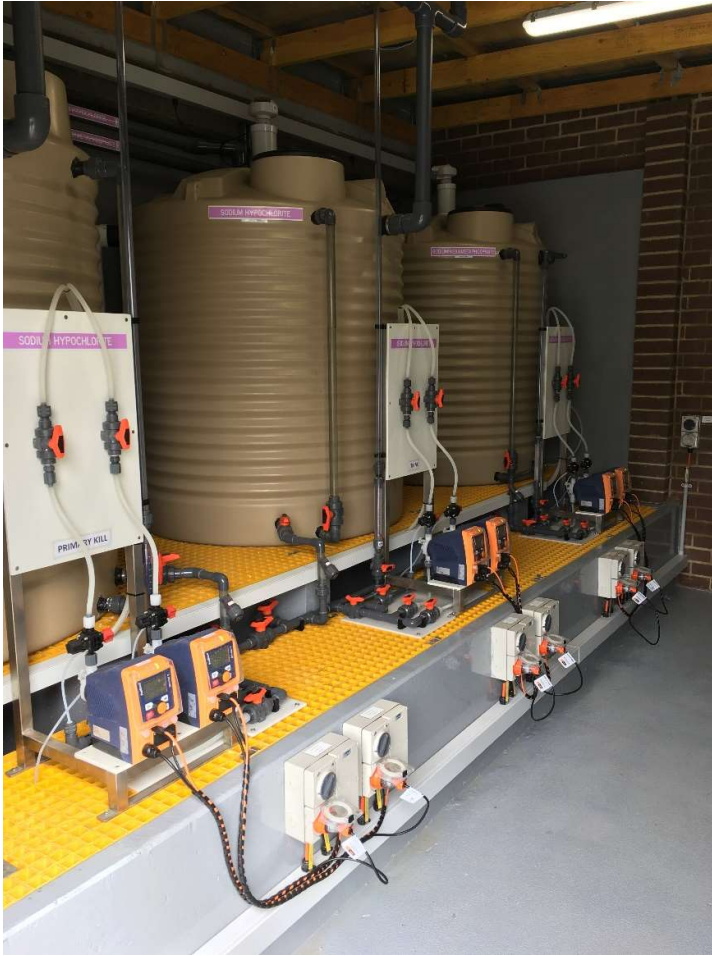
Figure 10: Heyfield water supply locality project – Chemical dosing system
