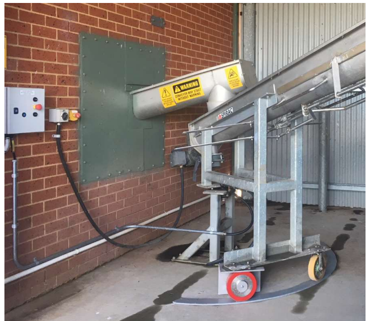
Figure 9: Warragul Water Treatment Plant – Sludge centrifuge tracking system Warragul Water Treatment Plant upgrade to sludge centrifuge tracking system to reduce worker manual handling and improve process control.
