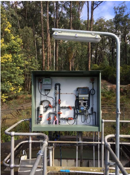
Figure 8: Maffra, Mirboo North and Warragul Water Treatment Plant – Streaming Current control unit Maffra, Mirboo North and Warragul Water Treatment Plant – Commissioning of Streaming Current Detector process control units to improve water treatment plant performance and reliability
