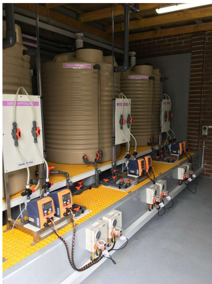
Figure 10: Heyfield Water Treatment Plant – Chemical dosing system
