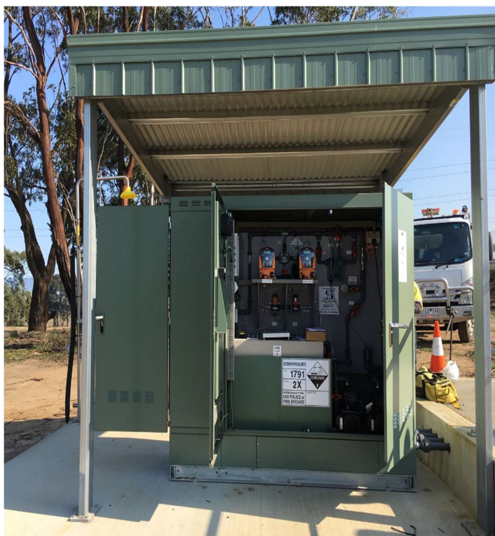
Figure 11: Morwell water supply locality Ridge Reservoir project – Chemical dosing system
