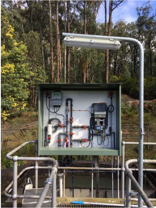
Figure 8: Maffra, Mirboo North and Warragul Water Treatment Plant – Streaming Current control unit
