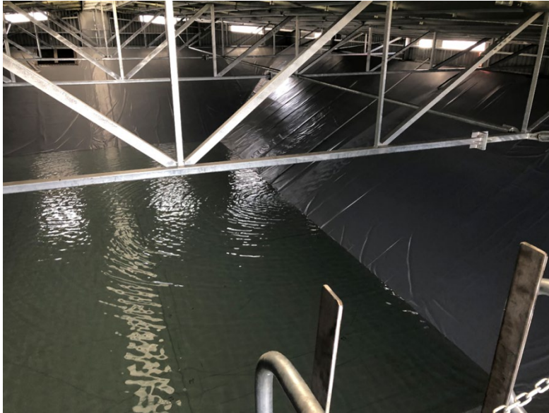
Figure 12: Neerim South Water Treatment Plant – Treated water basin cover and liner upgrade
