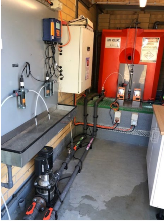
Figure 10: Jeeralang North water supply locality Ridge Reservoir project – Chemical dosing system
