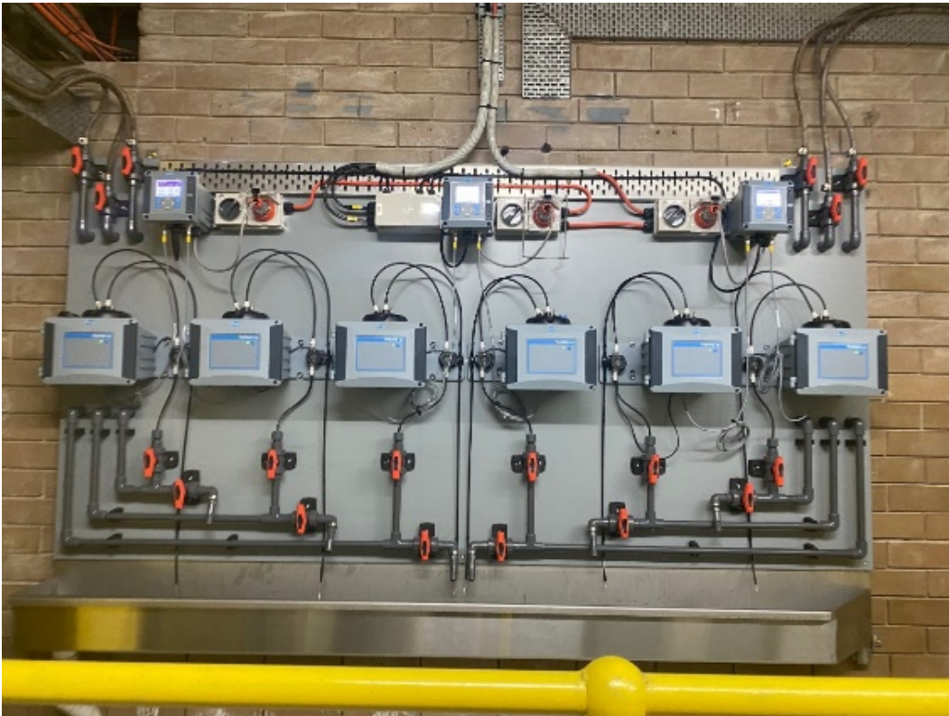
Figure 16: Filter outlet turbidity instrument replacements Morwell WTP
