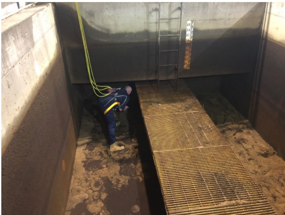
Figure 11: Scheduled manual cleaning of filter media at Morwell WTP
