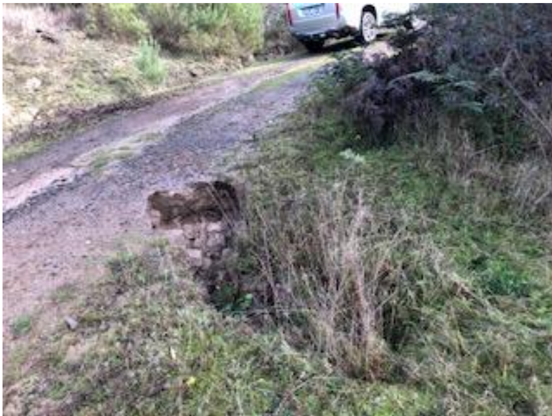
Figure 12: Assessing repairs required in the aftermath of the June 2021 Storm event in the Moondarra Catchment
