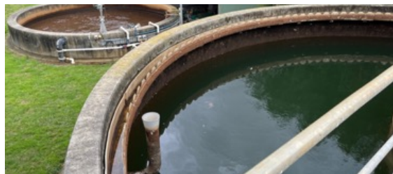
Figure 6 - The sludge clarifier at Warragul WTP which contained high level of MIB. Water from here is typically returned to the head of the plant for recycling.
